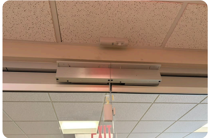
Mag-locks on double glass doors: exactly the kind of opening that needs permits and a fire alarm tie-in.
